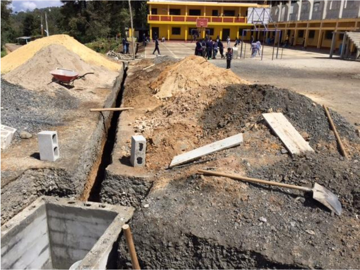
New Septic System for the entire learning center!
